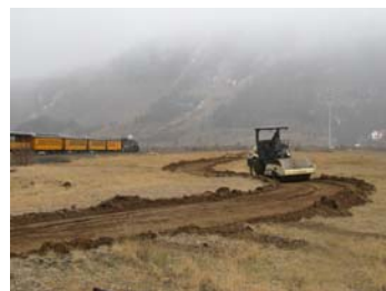
Many thanks to Pete Maisel and his construction crew for cutting the new DSNGRR trail in Fall of 2008!
